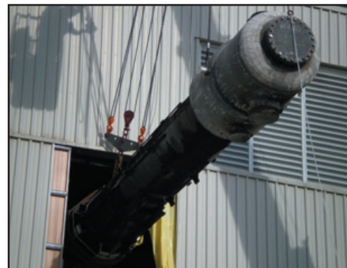
Strategic and experienced rigging was required to remove the existing bundles and install the new ones
