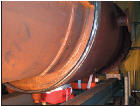
The heater to piping alignment and fit-ups, and zero-defect welding, improved the schedule by two days.
