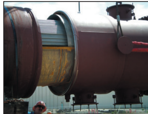
A 60" clamshell cutter was used (vs. grinding) to sever the shipping container from the replacement bundle
