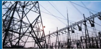
Transmission & Distribution Services
